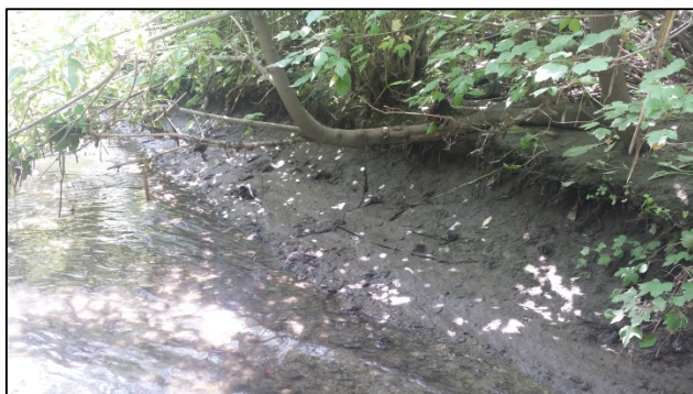
Photograph 5: Observed bank erosion at Black Creek; view at right bank of stream on July 8, 2015.
