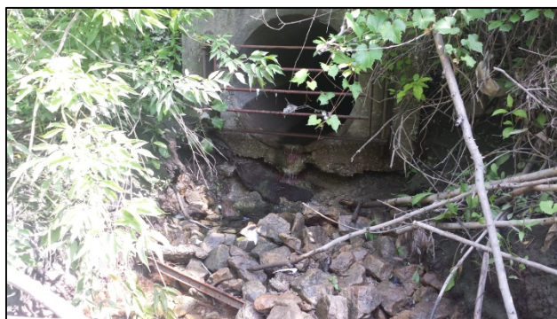
Photograph 4: Elevated stormwater outfall at Black Creek; view at left bank of stream on July 8, 2015.
