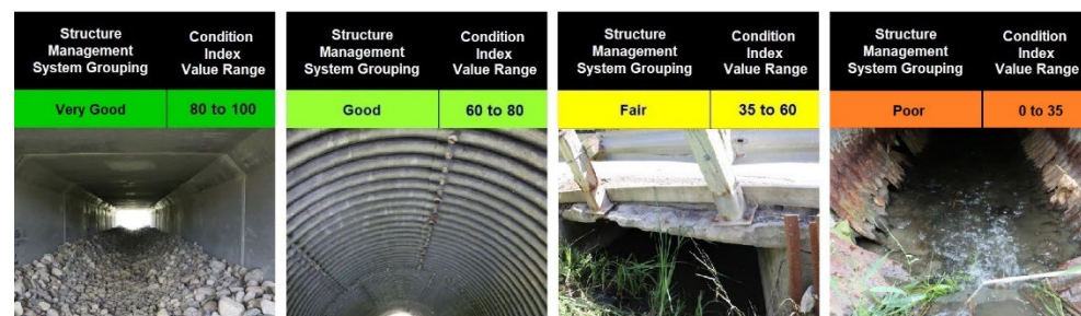
Figure 6-10: Images of Culvert Inspections Compared to Asset Management Condition Rating
