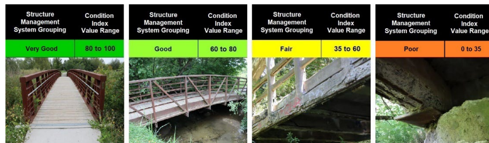
Figure 6-9: Images of Bridge Inspections Compared to Asset Management Condition Rating
