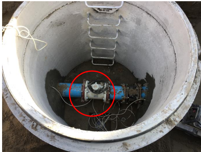
Water meter on water pipe within a chamber to measure leakage in a specific area
