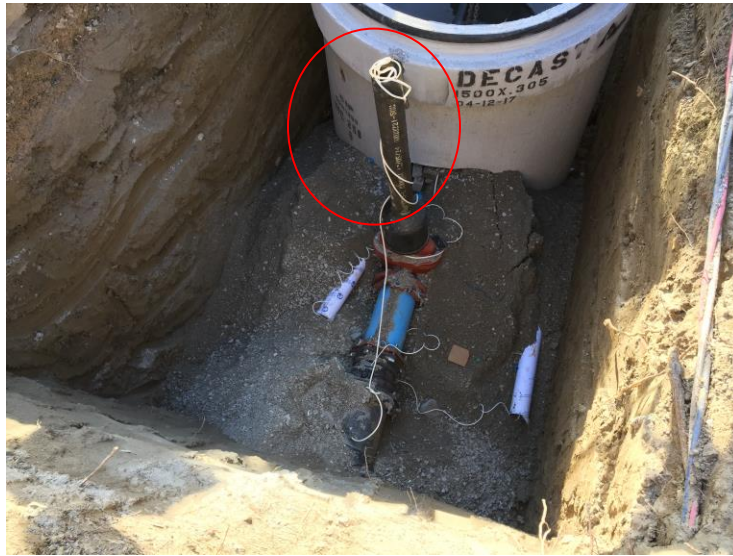
Anode Attached to Pipe Reducing Corrosive Effects
